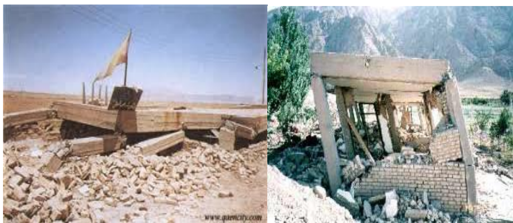
Figure 11. An example of damage to R/C frame buildings during the Ardakul earthquake
