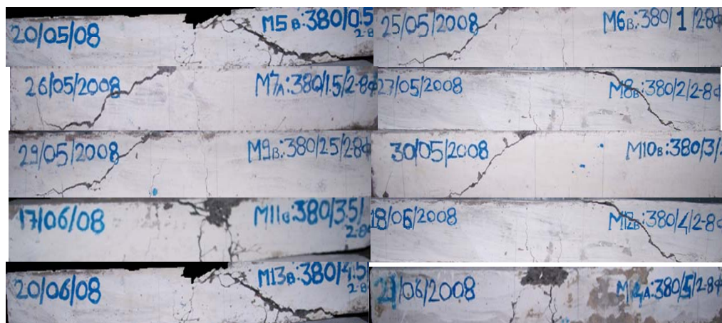
Figure 4. Failure pattern of beams with different fibre content
