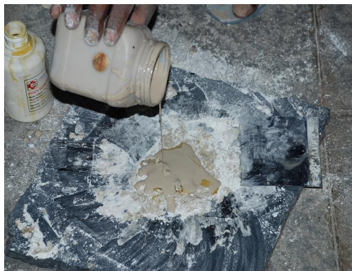
Plate 1. Mixing ESSEN base and hardener to fill groove and fix the PVC pipes
