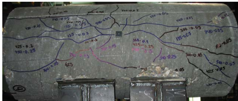
Figure 4. Crack pattern of specimen EB3 and dislocation around the support elements (bottom side view)
