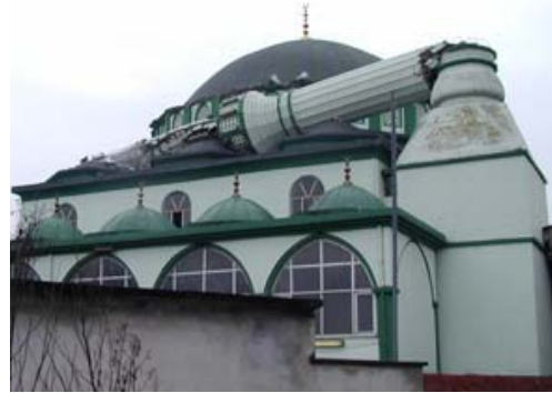
Figure 2. Collapse of minarets due to failures near the bottom of the cylinders
