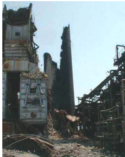
Figure 3. Remnants of failed stack
