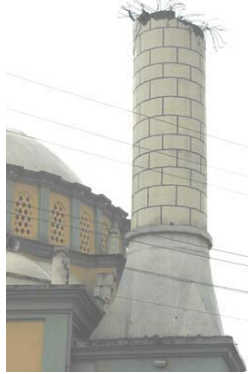
Figure 1. Damage to cylinder mid-height
