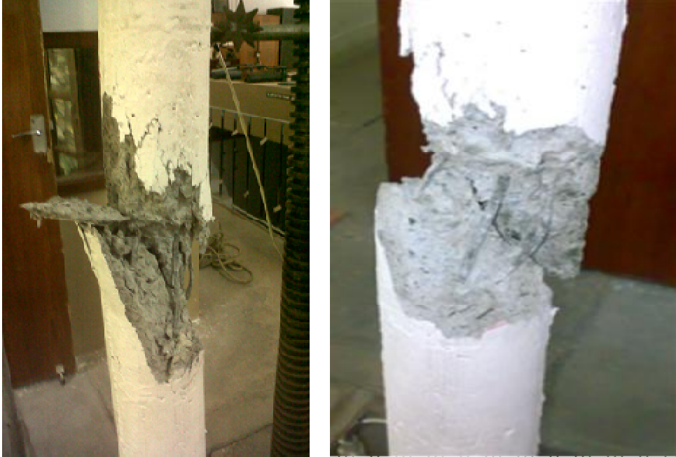
Figure 7. Failure pattern of G30 concrete column (typical)
