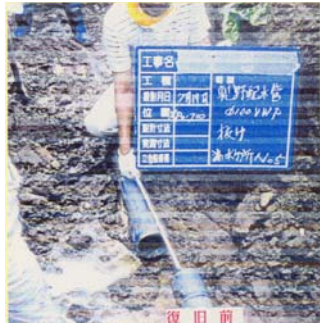
Photo 1. RR joint slip-out
